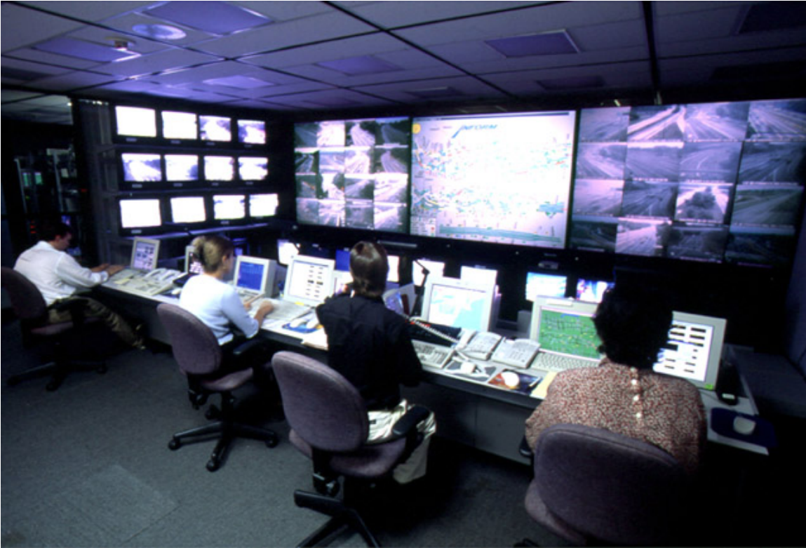
Figure 4-1. INFORM (Long Island, NY) Control Center.
