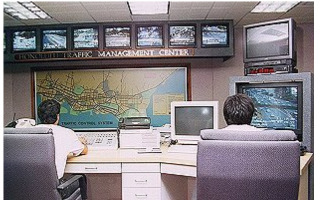
Figure 8-1. Traffic Management Center (TMC) (1).
